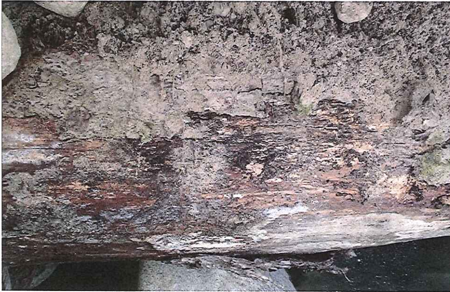
CK2210 Stringer crushing failure
