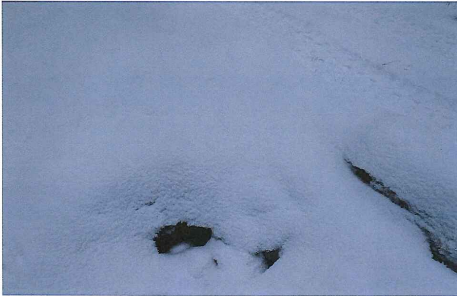
CK2210 Deck Scour
